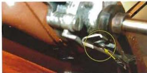
... and here the points, now open, which give earth (in closed position) to the wiper motor.
